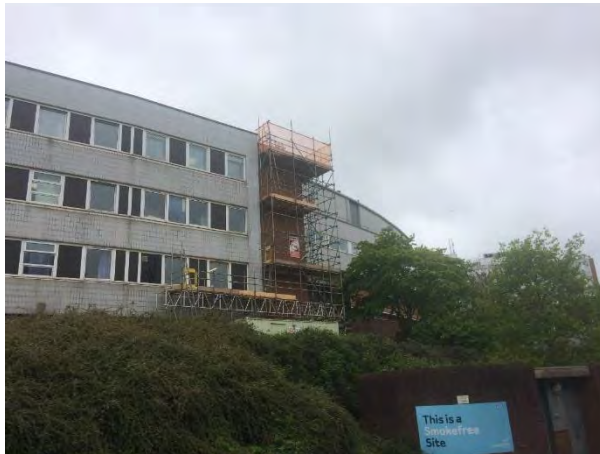
Figure 4-10- Image below: Dilapidated building housing office and clinical support services accommodation and storage
